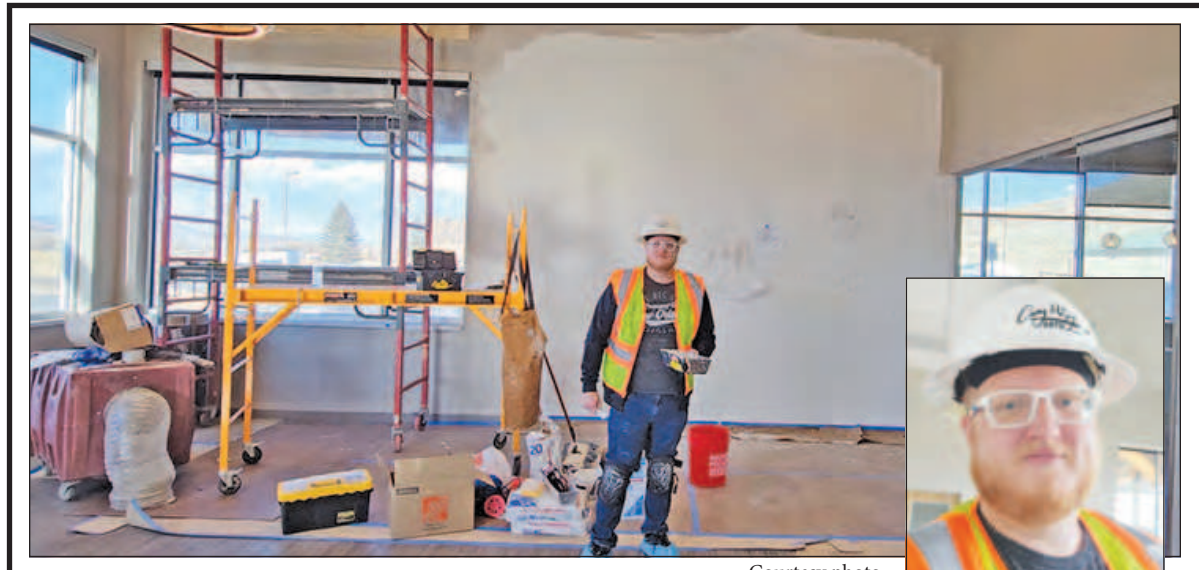
Courtesy photo Local artist Casey McCoy has been selected to showcase his talent as a drywall artist in the new Rio Grande Hospital wellness center. Casey McCoy
