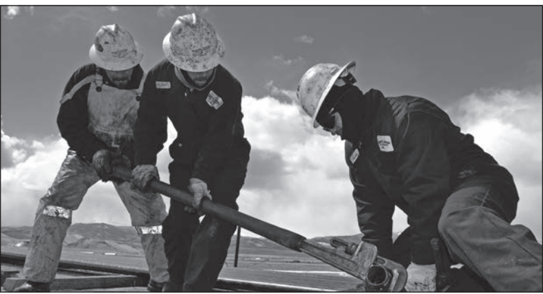
Workers disassemble piping used in the fracking process at the FLE drill site.
