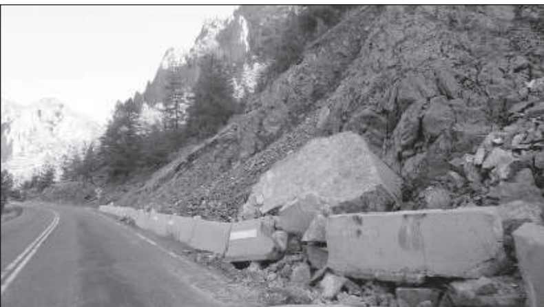
A large rock about the size of a small compact car fell onto Highway 149 during the evening of July 15, blocking the road.
