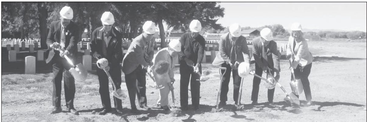
Turning the first shovels full of soil on the new Colorado State Veterans Center cemetery expansion are, from left, Reggie Bicha, executive director of the Colorado Department of Human Services; former State Senator Lewis H. Entz; Jay Bobick, chairman of the Colorado Commission on State and Veterans Nursing Homes; Maryann Terry, Colorado Commission on State and Veterans Nursing Homes; Youlon Savage, chair of the Colorado Human Services Board; State Senator Larry Crowder; Robbie Robinson, chair of the Colorado Board of Veterans and Military Affairs; and Viki Manley, director of the Office of Long-term Care in the state Department of Human Services.
