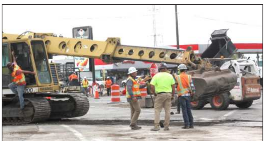
An improvement project is underway to improve the intersection of US Highway 160 and CO Highway 17. Upgrades to the intersection include a new traffic signal that will replace stop signs currently at this location.
