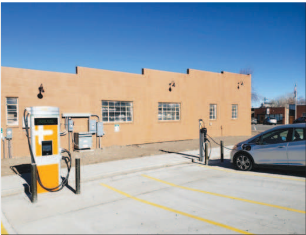
Del Norte charging station.
