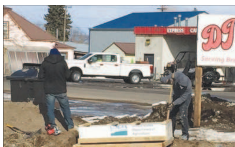
Bridge work began last week, the final steps for completing the Safe Routes to School project in Center.
