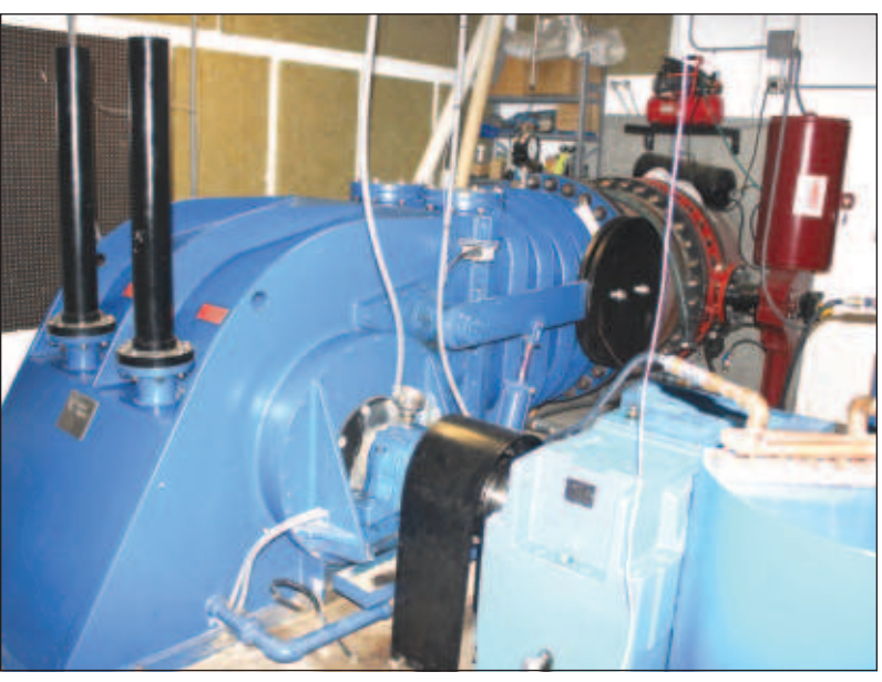
The single-phase, crossflow turbine generator operating on Humphreys Ranch, is affectionately called "Miss O", named after the ship "Octavia" that brought the massive unit to the United States from where it was built in Italy by a company specializing in three-phase generators. The generator can produce up to 300 kW which could provide power to 200 homes, according to SLVREC. On Saturday, it was producing 100 kW.
