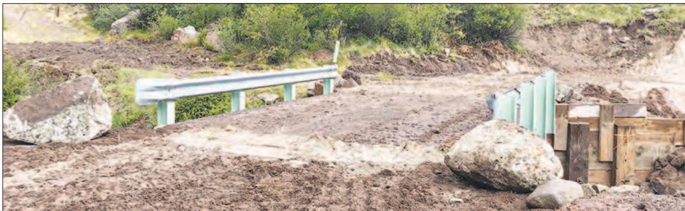
Bridge repairs have been completed allowing for the road to Continental Reservoir to reopen.
