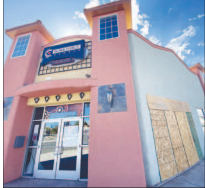
The Colorado Workforce Center located at the intersection of State Avenue and Fourth Street, suffered damage on Oct. 8 during a car crash when a Honda Civic careened into the building. The building is currently closed.
