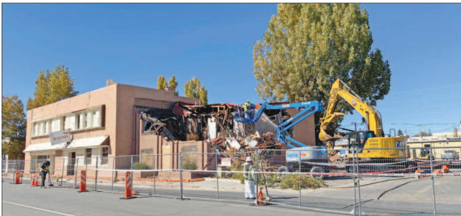
Work crews began demolishing the derelict Walsh Building on 6th Street in Alamosa on Tuesday. The demolition of the building owned by the City of Alamosa is expected to take several days.
