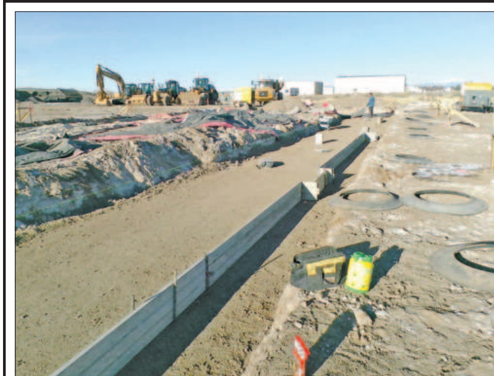
Photo Courtesy Will Hickman, San Luis Valley Regional Airport Work continues on the Snow Removal Equipment building under construction at the San Luis Valley Regional Airport.
