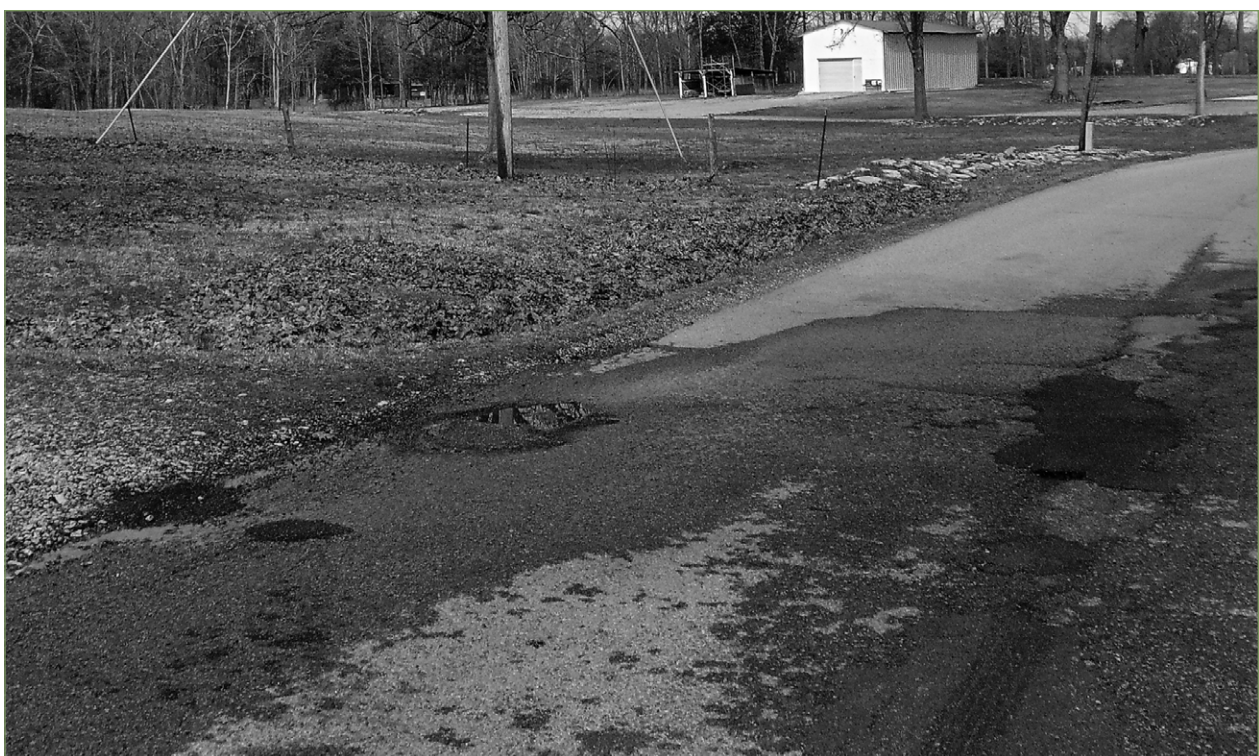
Despite some patch jobs, El Bethel Road off 41A is still a bumpy ride for residents.
