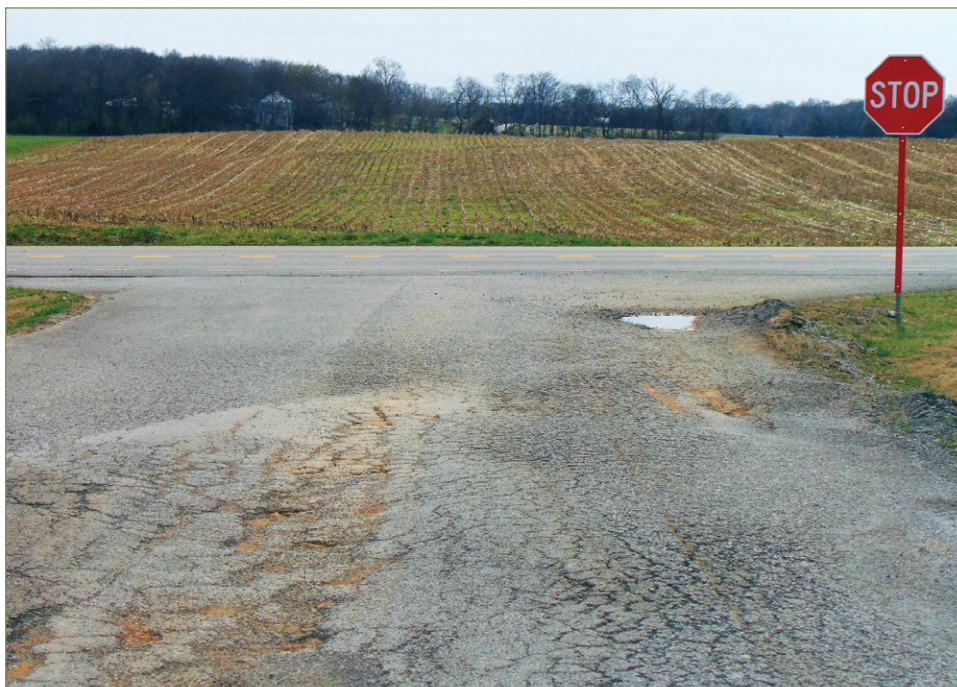
Residents at the intersection of Unionville-Deason Road and Tyler Drive have a bumpy ride daily right now as they ride over potholes and crumbling asphalt. T-G Photo by Zoe Haggard
