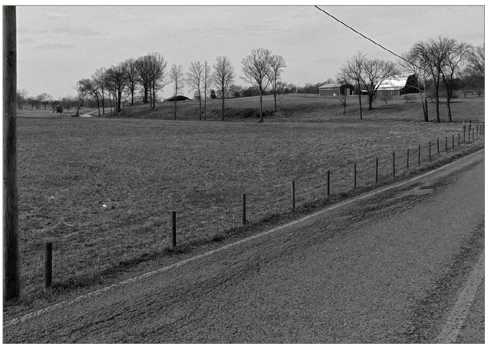
Old Nashville Dirt Road is beginning to resemble an actual dirt road in some spots with sunken asphalt.
