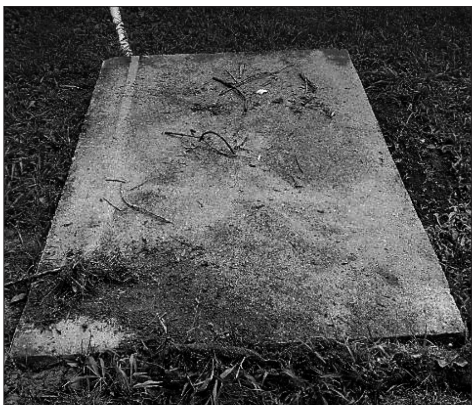
After Kasinger filed a zoning complaint for the open septic tank in their yard, the landlord put a concrete cap over the plywood. But Kasinger said you can still smell the toilet waste, especially when it rains.
