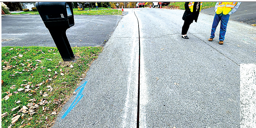
This two-inch-deep "microtrench" was installed by Archtop Fiber last year as a test along a residential street in Saugerties. The cut is pictured as it is about to be paved over, sealing in the cabling.
