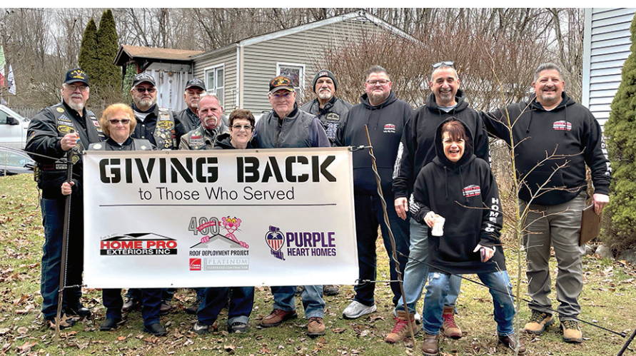
As part of Owen's Corning Roof Deployment program, a US veteran received a cost free roof. Home Pro donated their labor and covered disposal costs. Home Pro does several Veteran roofs per year.
