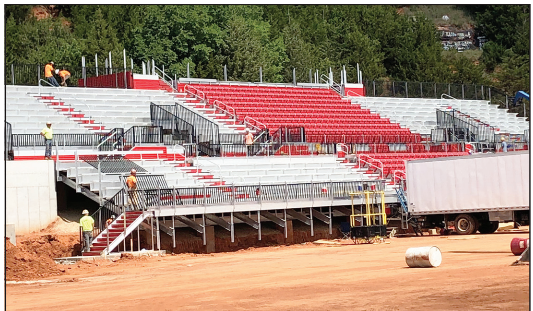
• Photo provided Taking a stand The home stands at Conger Field have begun to take shape this past week as construction continues in preparation of the September 6 home opener with the Lindsay Leopards.
