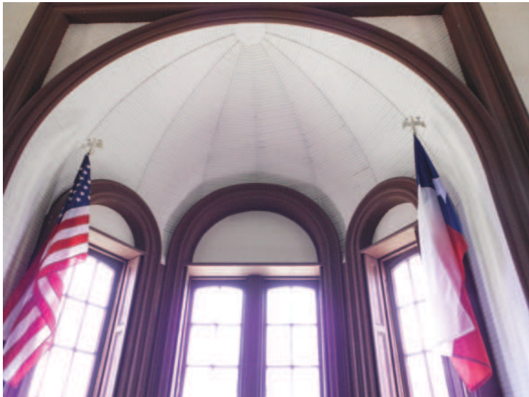
The ceiling above where the judge sat is filled with sand to act as a fire suppressant if the boards were to catch fire.
