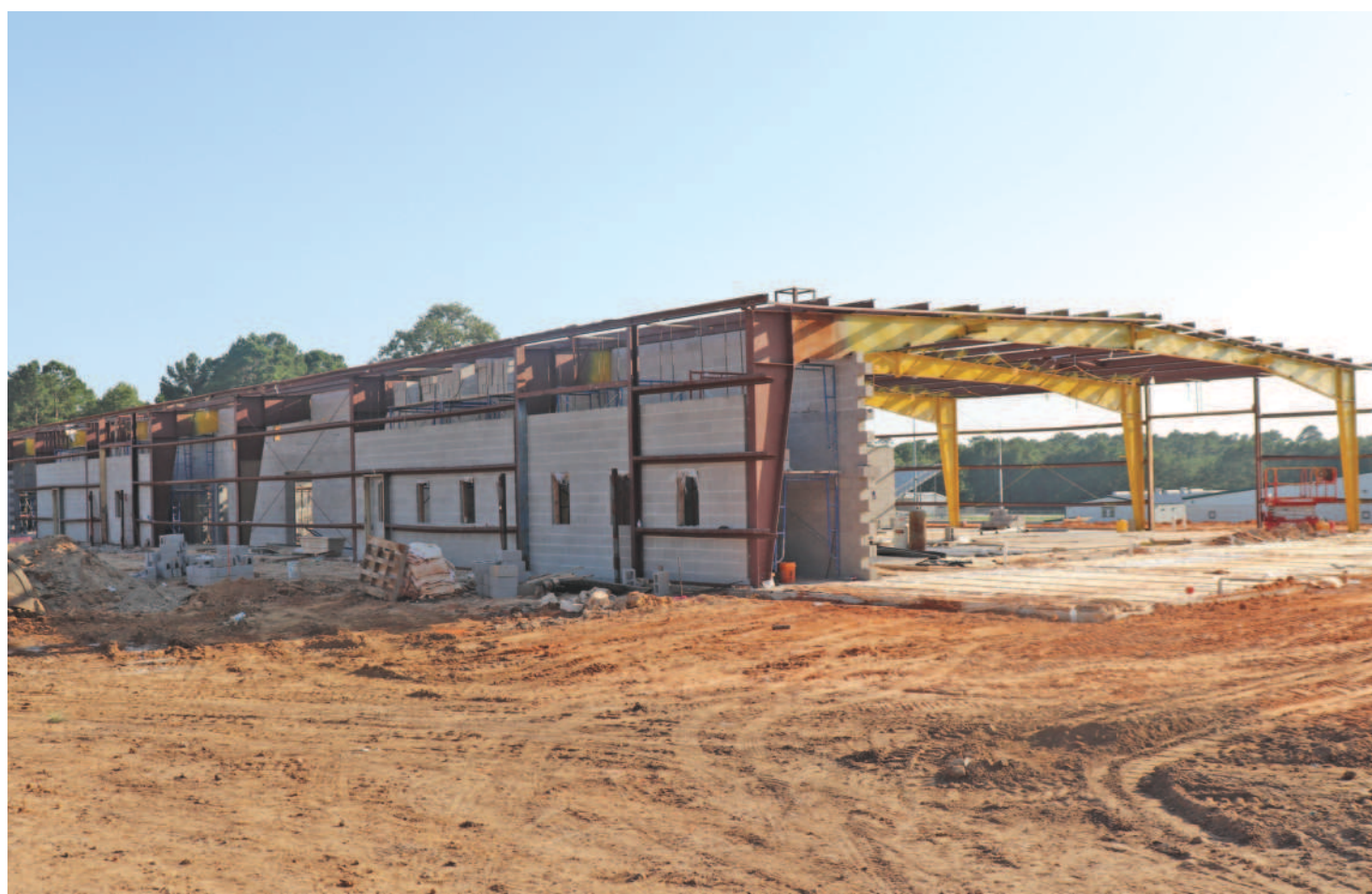
Progress happening – The new CTE building on the campus of Woodville High School is taking shape. CHRIS EDWARDS | TCB
