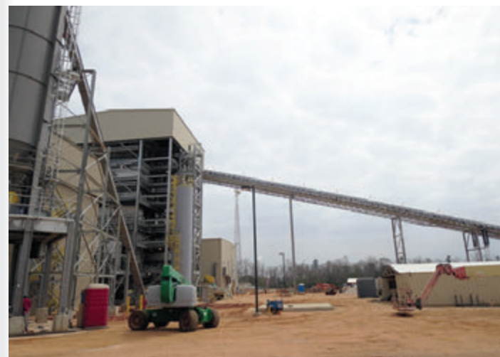
East Texas Electric Cooperative's new Woodville Renewable Power Facility, which is nearing completion, will produce 49 megawatts of clean, carbon-neutral electricity close to home for Cooperative members. It will also diversify ETEC's generation portfolio for its distribution cooperative members, including Sam Houston EC.
