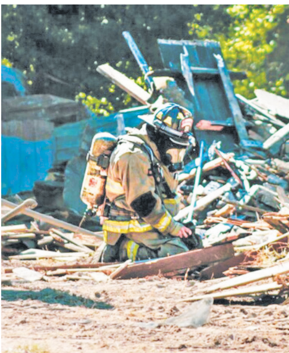
A Trinity firefighter assisted Centerpoint in sealing a gas leak that developed at a job site. COURTESY PHOTOS
