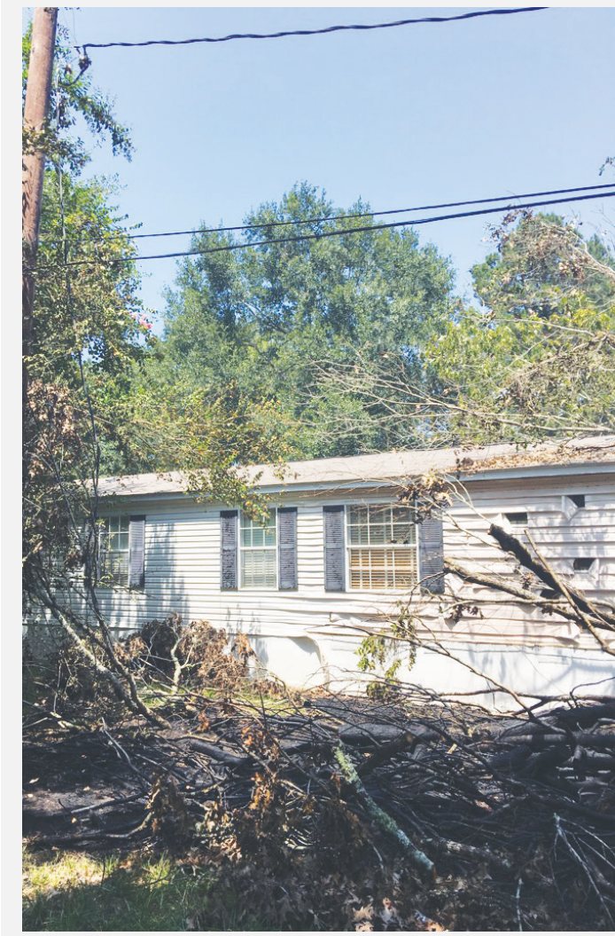
The siding of a residence in the Westwood Shores subdivision was melted from the heat of a blaze that broke out when a downed power line ignited debris on the ground. COURTESY PHOTO
