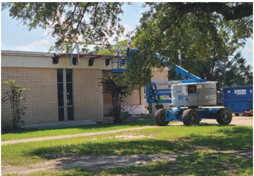
All campus exteriors will receive a facelift, as work begins on the high school. PHOTO BY BRIAN BESCH
