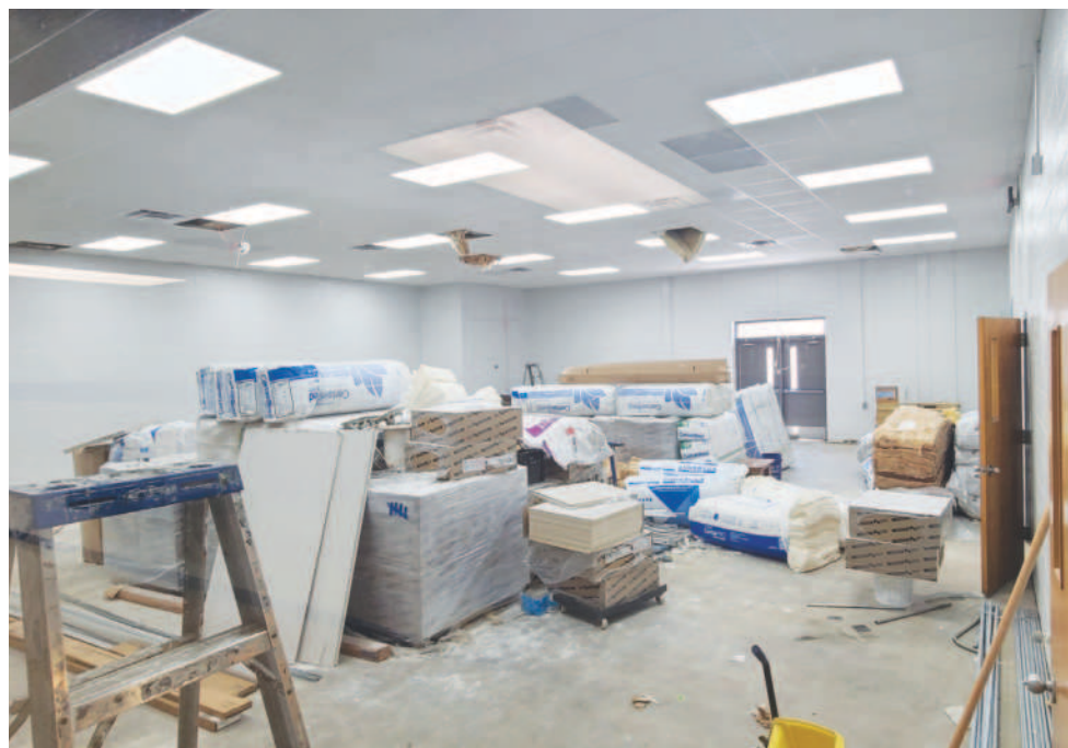
The junior high cafeteria will feature upgrades in plumbing, drainage, cooking and cleaning equipment, serving lines, and undergo an expansion. PHOTO BY BRIAN BESCH
