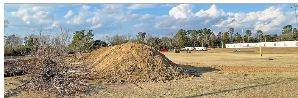
Dirt is being cleared in preparation for construction of the FEMA gym/shelter.
