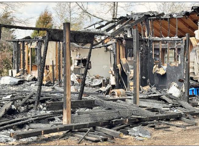
This house on Curtis Drive was destroyed by fire Feb. 4.
