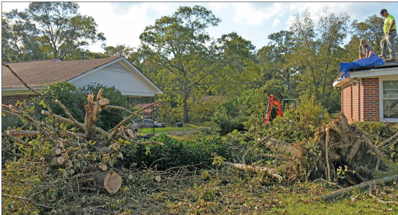
S.C. Baptist Disaster Relief crews work to cut trees that fell on this home on Winton Street in Barnwell and place a tarp on a damaged part of the home's roof following Hurricane Helene.
