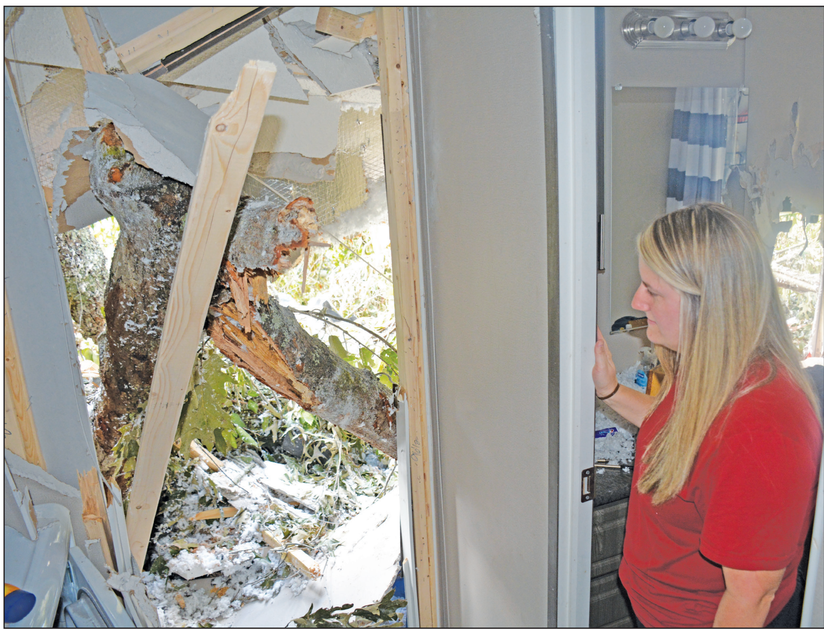
Victoria Creech stands in the doorway of a bathroom in her Fellowship Road home as she looks at what used to be her son Caden's bedroom. The bedroom was obliterated after Hurricane Helene brought several trees down on it.
