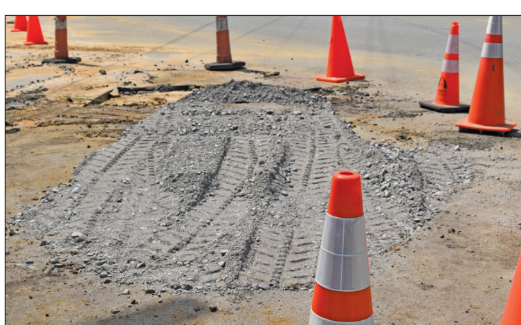
Part of road buckled at the intersection of Elko St. and Springfield Rd. as a result of consecutive main water line breaks.
