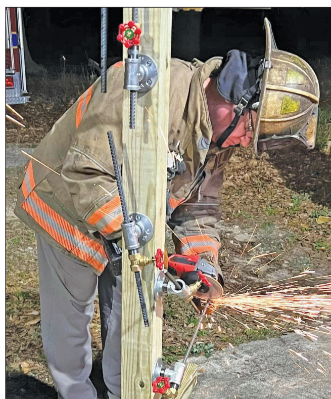
A Williston firefighter cuts through a prop using new equipment the department received through ARP funds. Contributed Photo
