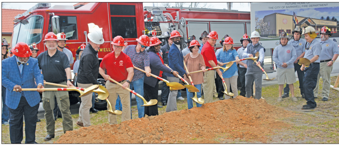
Leaders from the City of Barnwell join with S.C. Sen. Brad Hutto, Rep. Lonnie Hosey, and contractors to break ground on the new Barnwell Fire Department. It's expected to open next year.
