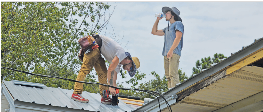
Hunter Harris, left, works on a roof while his brother Joshua, right, hydrates himself. During last week's heatwave, Hunter had to stay home for two days due to heat exhaustion.
