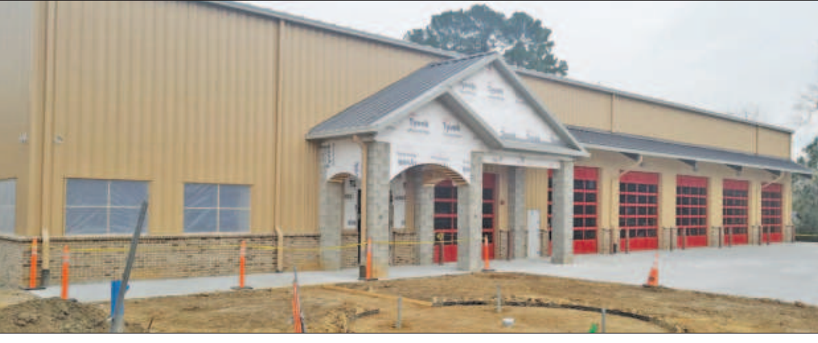
See BOND, 10A The new fire station for the Barnwell City Fire Department is nearing completion.
