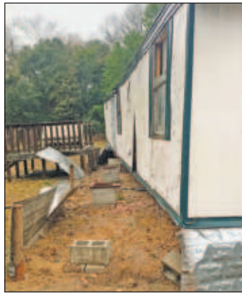
This home on Nick Street in Blackville was ripped from its foundation. Contributed Photo
