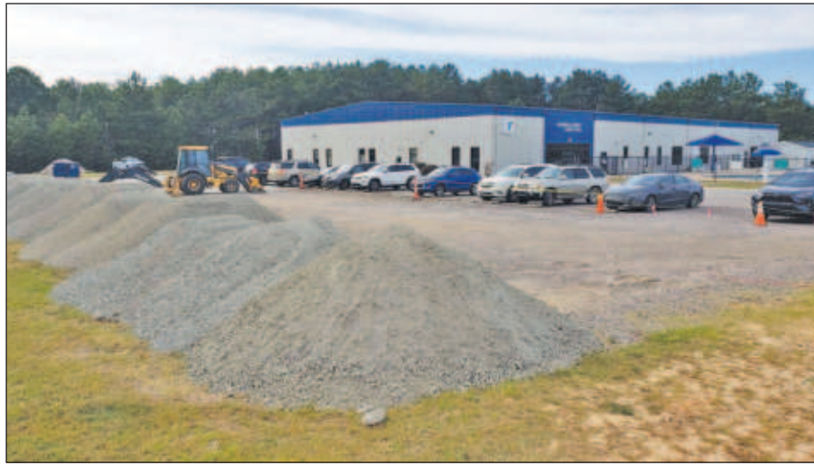
The piles of gravel being used as site prep represent the location of the four upcoming pickleball courts at the Barnwell County YMCA. Courtesy: Barnwell County
