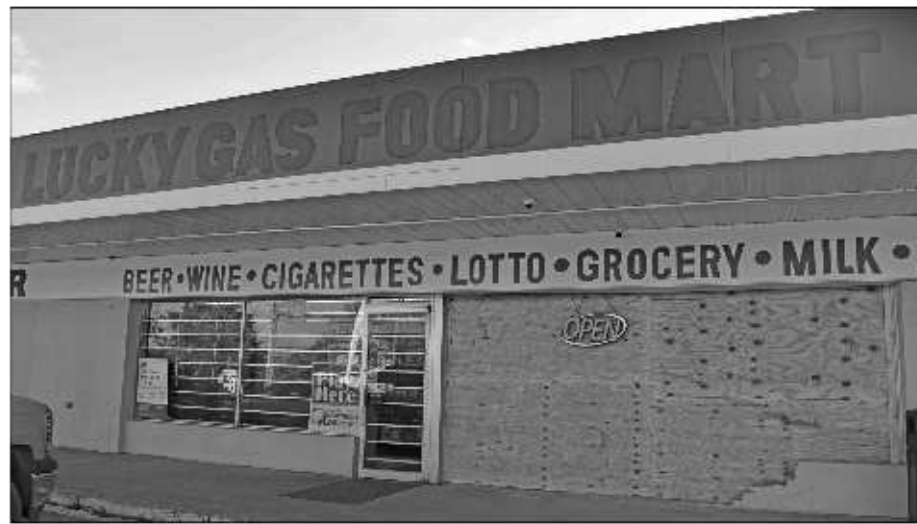
The front window of Lucky Gas Food Mart in Williston remains boarded up more than one month after a car plowed through it. Alexandra Whitbeck / Reporter
