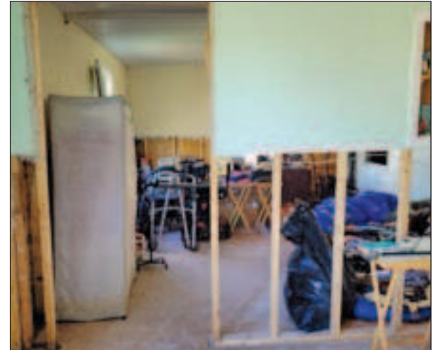
A stripped wall in a Florida home impacted by the hurricane. The Church of Jesus Christ of Latter-day Saints helped hurricane victims.
