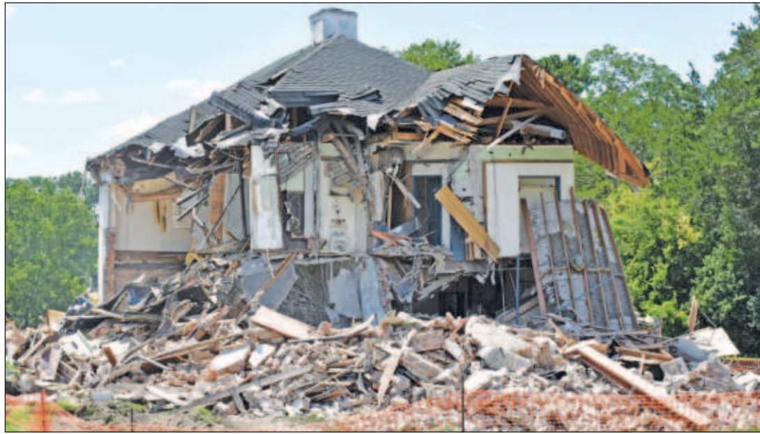
Only photos and memories remain of the old jail/sheriff's office building after the dilapidated structure was torn down in July.
