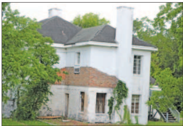
Exposed brick can be seen on the old dilapidated sheriff's office/jail.
