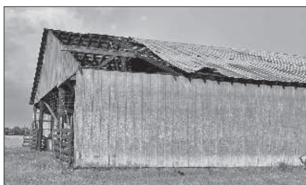
This shed in the Long Branch community was one of several structures damaged last week by a microburst.
