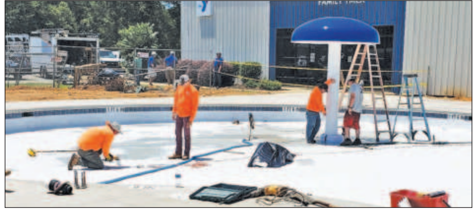
Workers put the final touches on the children's pool at the YMCA aquatics center in Barnwell. The center officially opens to the public on June 11.
