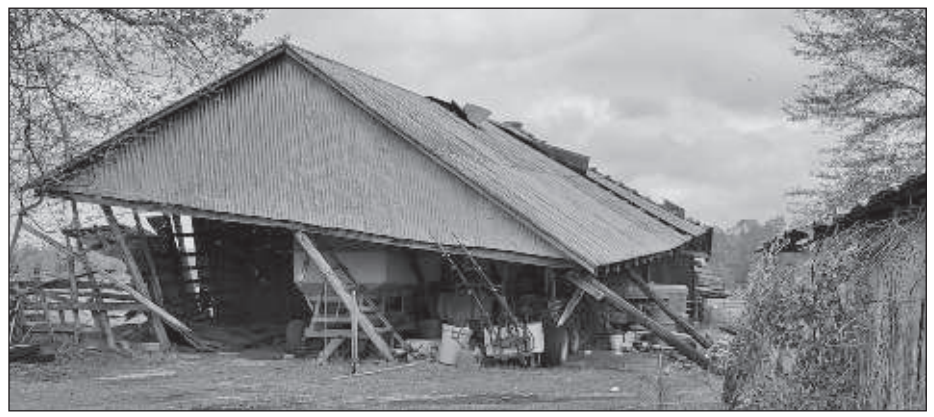
This barn on Amanda and Jonathan Croft's property in Bamberg County was destroyed.
