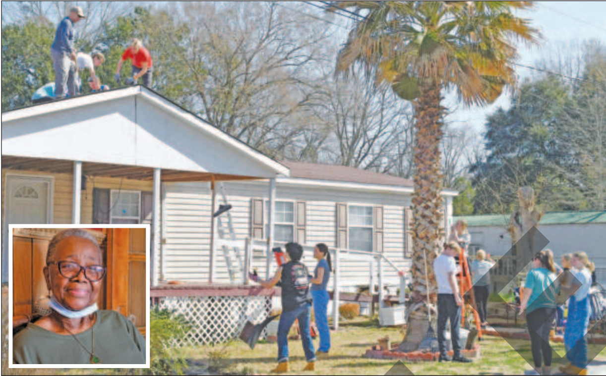
A new roof and front stairs were provided by teen volunteers from Connecticut as part a revitalization project. Homeowner Gloria Harvey (inset) called the work a "blessing".
