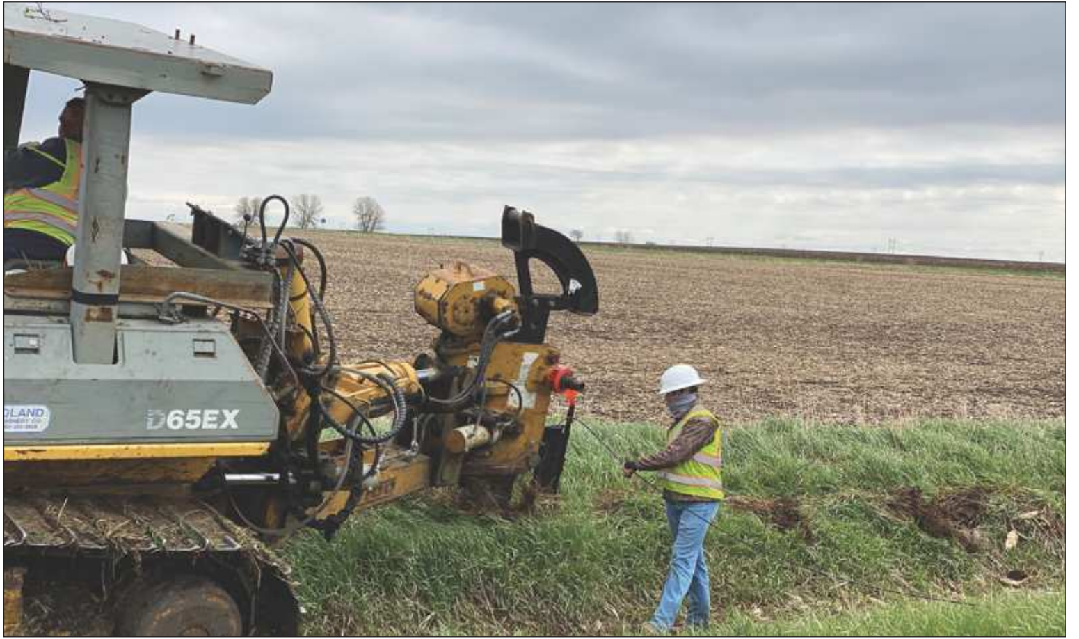
Kenny Richison and Bailey Hamm with Telcom Construction out of Clearwater, Minn., plow in cable and feed the fiberoptics line into the ditches southeast of Flandreau last week.
