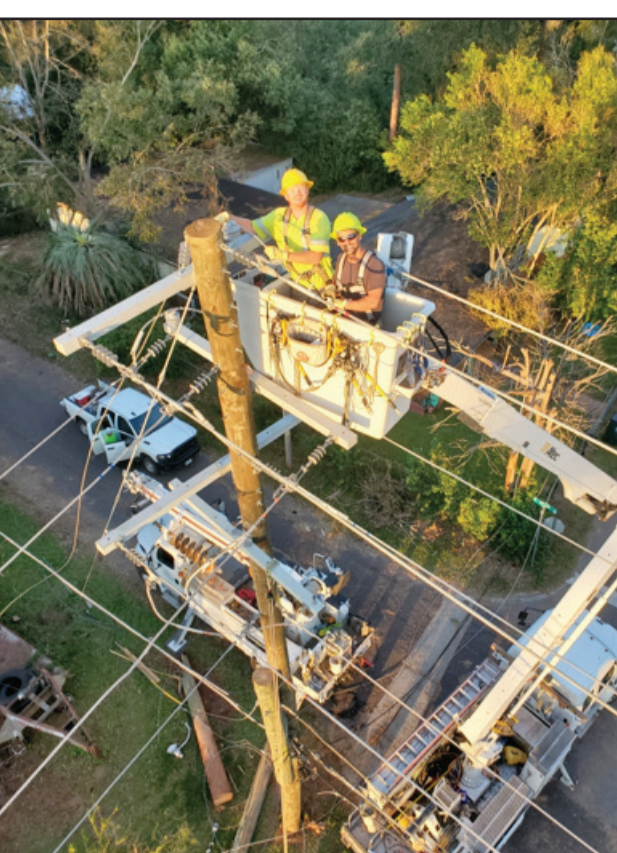
Linemen Jimmy Turcato, Todd Johnson and Casey Howard traveled to Georgia on Sept. 25 and returned Oct. 7. They spent time in Jackson, Elberton and Douglas, Georgia, working to restore power for residents. On Wednesday, Oct. 9, RMU sent another crew of four on a similar trip to Lakeland, Florida to assist in the aftermath of Hurricane Milton.
