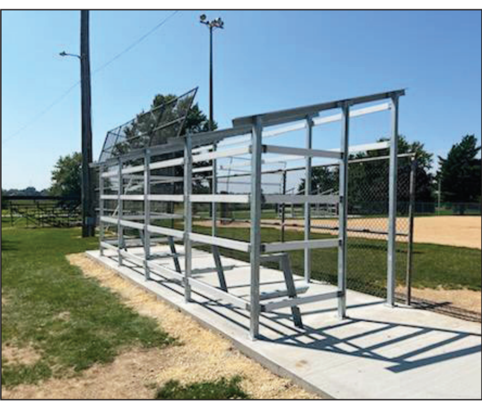
Dugout construction starts in Polo The Polo Lions Club started the construction on the dugouts at Westside Park on the morning of Saturday, Aug. 24. (Courtesy photos)
