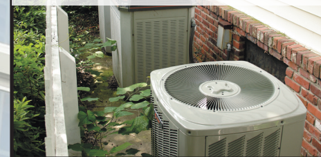
HEATING AND COOLING
