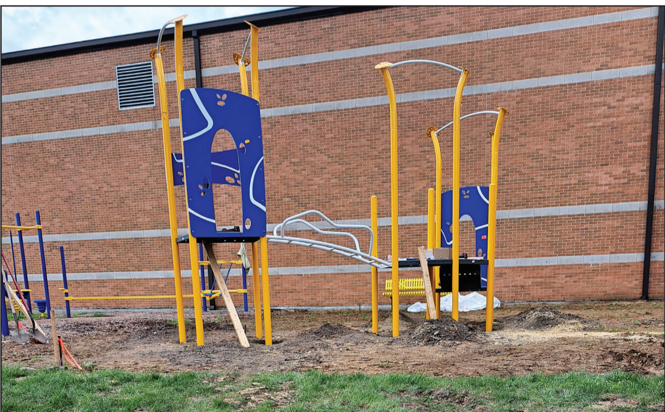
Polo Lions Club installs new playground equipment The Polo Lions Club was asked to put the new playground equipment up at Polo Centennial Grade School. The Lions Club started the work on July 5, also worked on July 6 and finished on Saturday, July 13. Each photo was taken to show where they finished on each day. Thank you to all the Lions members that worked on the project and they are: Mark Ebert, Mark Bocker, Nate White, Jim Adams, Keith Chesnut, Aaron Miller, Winton Bocker, Dustin Vock and John Deuth an also thank you to Brandt and Hayden Eastman for working on the project. (Courtesy photos)
