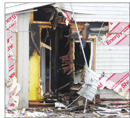
The home suffered at least $50,000 in damage from the fire. (Brad Jennings photos)
