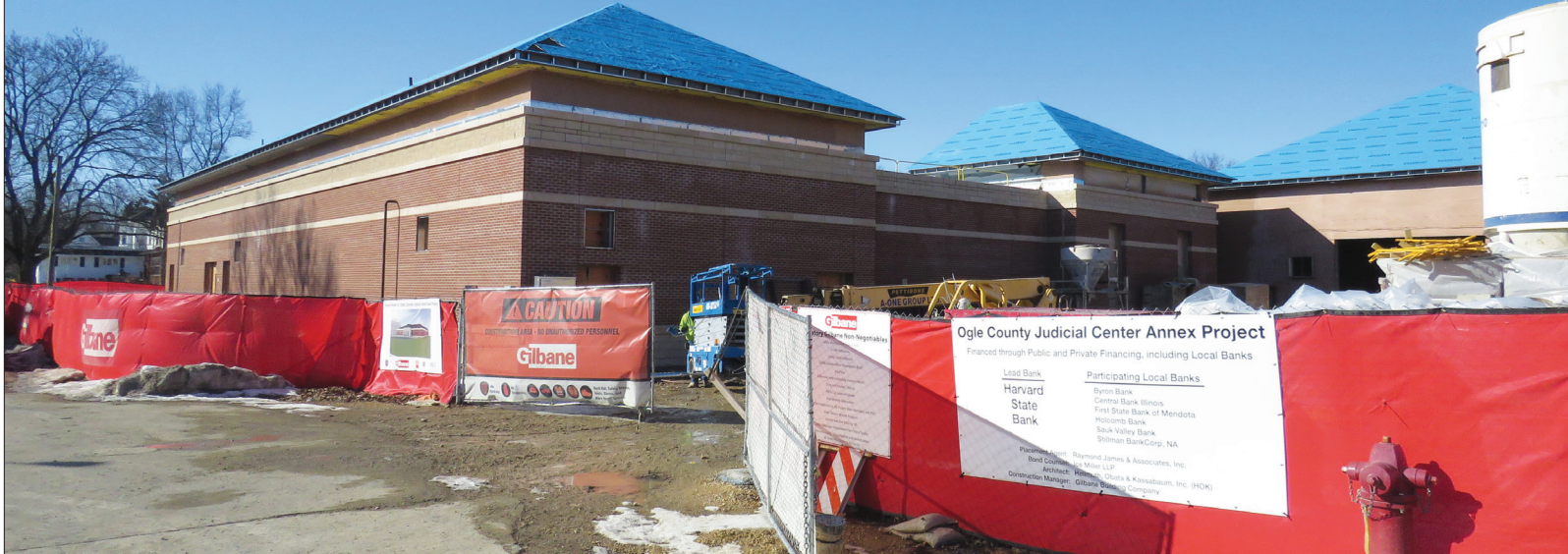
The roof on the new Judicial Center Annex in Oregon will go on this spring, as work inside the building continues. (Brad Jennings photo)
