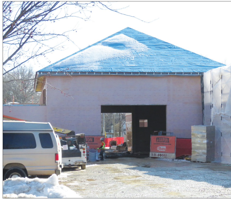
This Sally Port will connect the new jail to the Judicial Center to move prisoners safely to court. (Brad Jennings photo)
