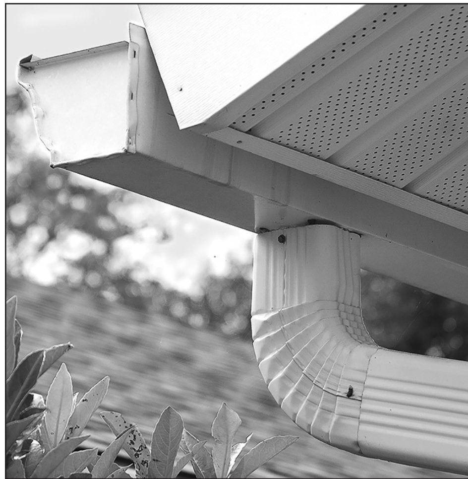
Compromised gutters can contribute to water issues in basements and adversely affect a home's foundation.
