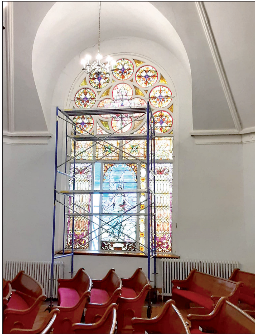
Scaffolding is in place to restore a stained glass window at First Presbyterian Church in Mendota thanks to support from church members, businesses and the community. (Photo contributed)
