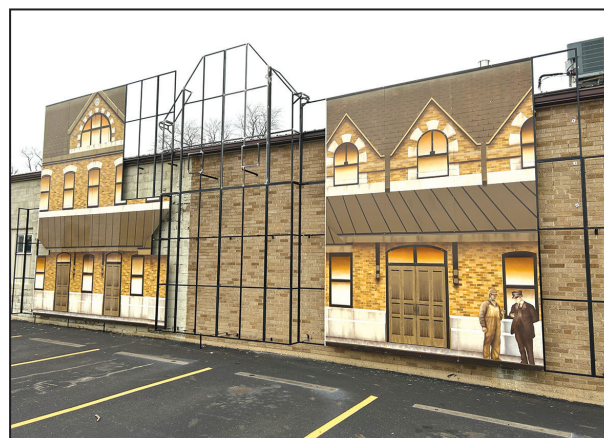
Installation of the “Raising the Depot” art mural as part of the Silo Pathways Countryside Public Art Tour is underway in downtown Mendota.
