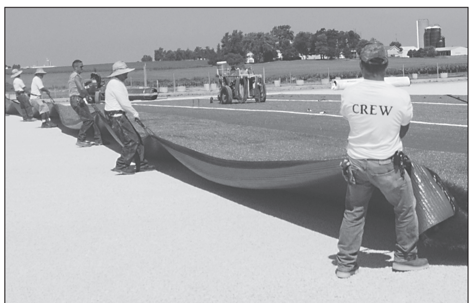
Mendota High School's new athletic stadium begins to "go green" on Friday, July 15, 2011, as workers from Extend Across the Field process laying artificial turf. The turf is laid in strips that extend across the field. Each strip is laid face down on top of the preceding one, the two are sewn together by machine on the underside and then unfolded. The 2023 Board of Education estimates that within the next five years, the track around the stadium will need resurfacing, and another estimate is for the turf replacement, and that should occur within the next seven to nine years.
