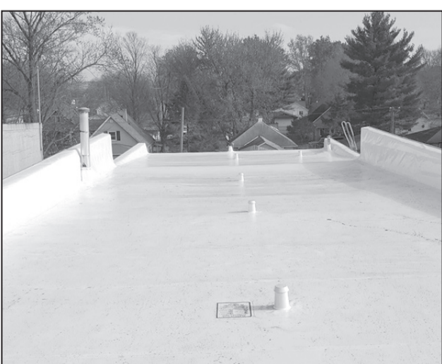
Northern Illinois Seamless Roofing, Inc. specializes in flat and low slope commercial roofing by installing the Duro-Last family of roofing systems. Duro-Last is the world's largest manufacturer of pre-fabricated single-ply roof systems. This system is ideal for any flat or low-slope roof.
