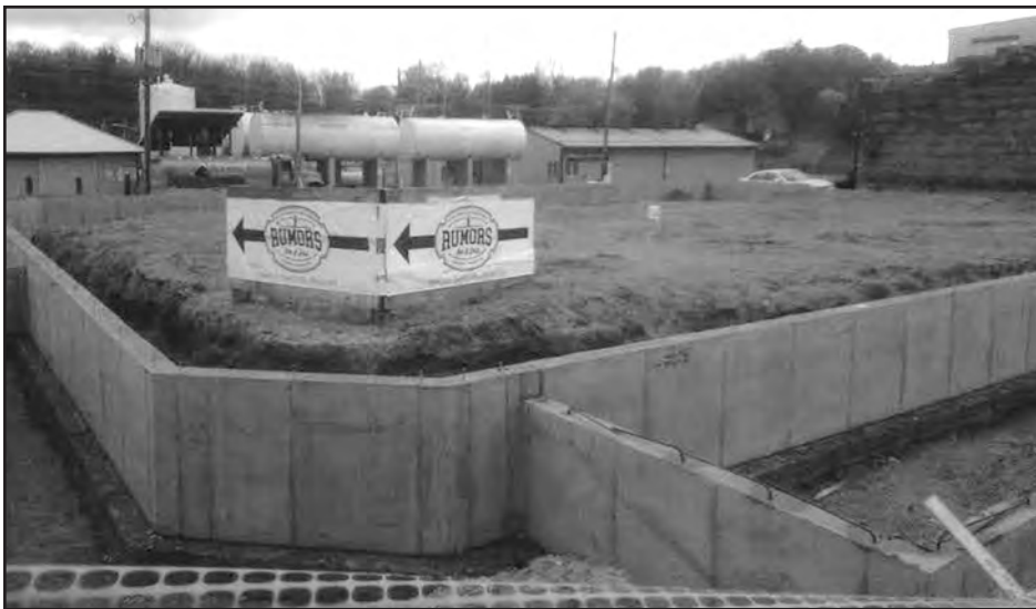
Construction on the new Rumors building has begun. The footings are now in place.
