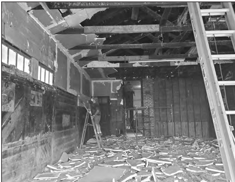
The entire inside of The Goodhue Depot needed to be torn apart and cleaned out. Most of the flooring was too damaged to save but the rest of the woodwork, the chimneys and doors were salvaged.
